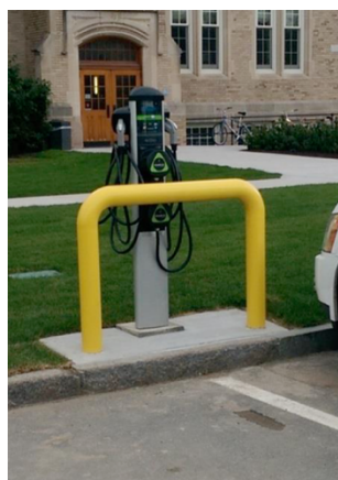
Figure SEQ Figure \* ARABIC 18: Tire stops used for EVSE protection (Source: Energetics)
